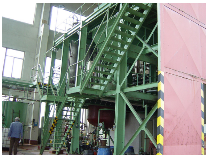
Fig. 9. Part of the device for the industrial trial (KORTAN Company, Hradek nad Nisou).
